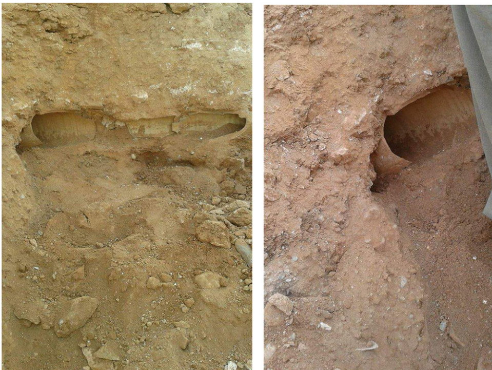
Figure 28. The destruction of ceramic drainage channels due to the digging work of a bulldozer (photo taken by a volunteer team member on 12 September 2015).
